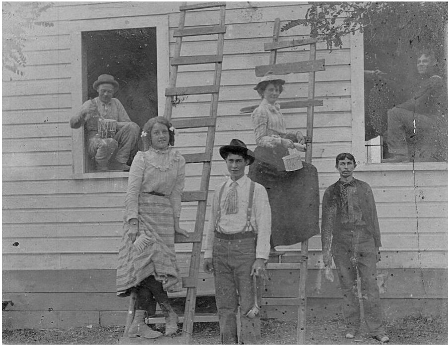
Painting the school, Hayfork Elementary 1898-1902. Left to right: Unidentified, Ella Vanderhoff (on ladder), Pindar Hailstone and John Kelley, others are unknown. Photo collection of Henry Meckel.
